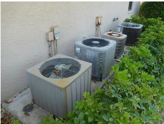
TYPICAL AIR CONDITIONER UNITS
